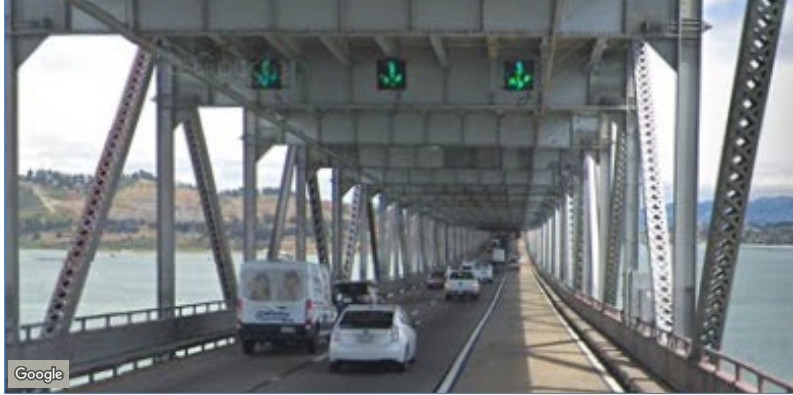
Figure 2-15: Electronic Lane Control Signs on Lower Deck
