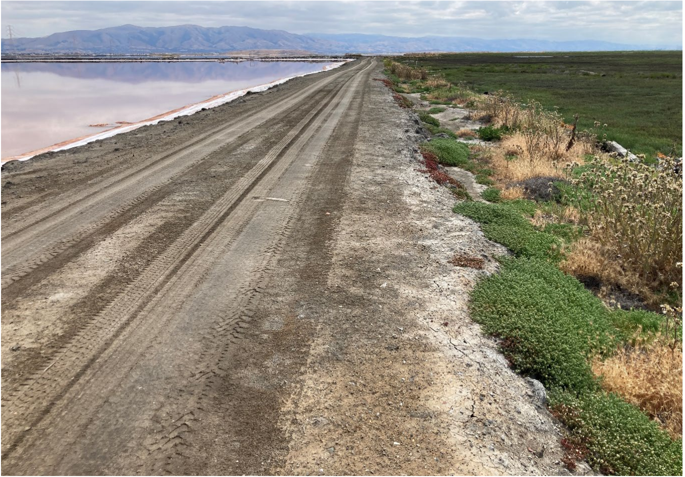
Photo 8. The outboard berm of Pond P2-12. It is drivable only during dry weather.
