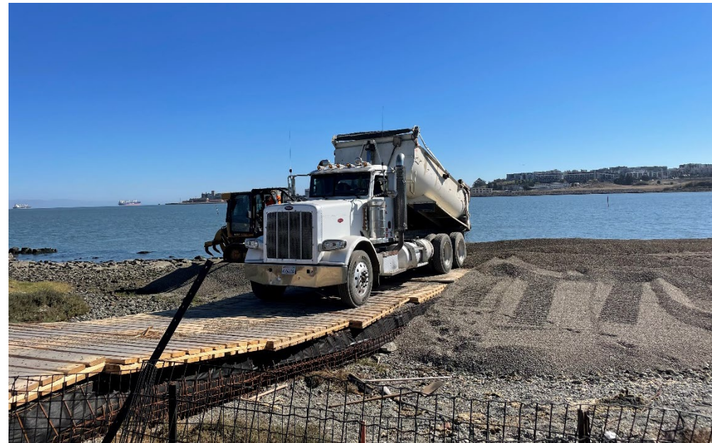
Gravel placement at Heron's Head Beach in San Francisco (Port of SF)
