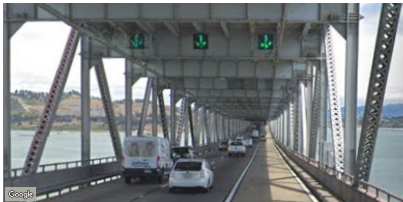
Figure 2-13: Electronic Lane Control Signs on Lower Deck
