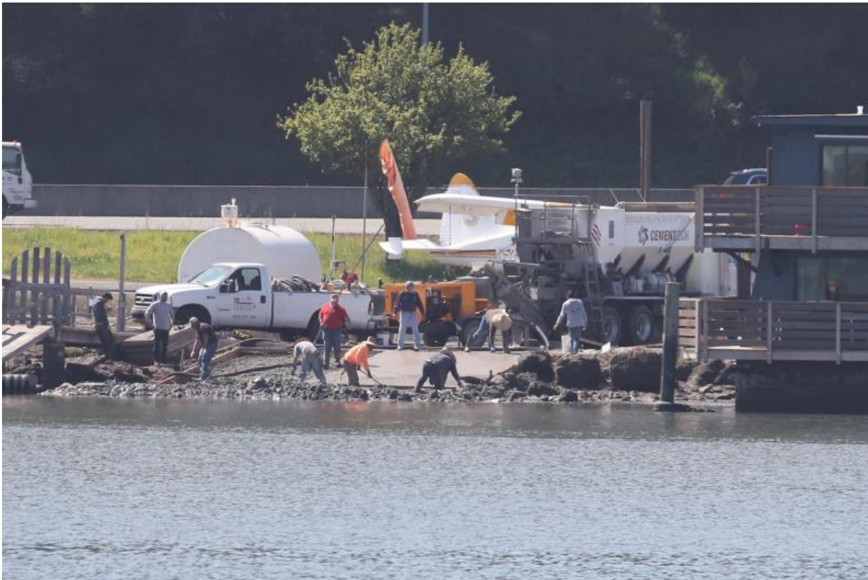
Exhibit 24C. March 14, 2022. Photograph 2 depicting unauthorized excavation and rebar and concrete ramp construction.
