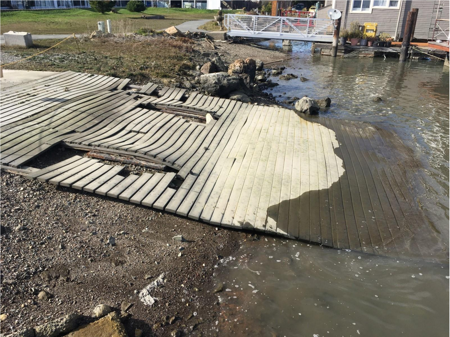
Exhibit 24A. January 31, 2020. Staff photograph depicting water access ramp before its unauthorized reconstruction in March, 2022. RED EXHIBIT 0
