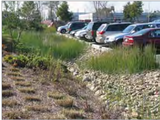
Stormwater runoff from the parking lot goes into this bioswale before draining into Elmhurst Slough
