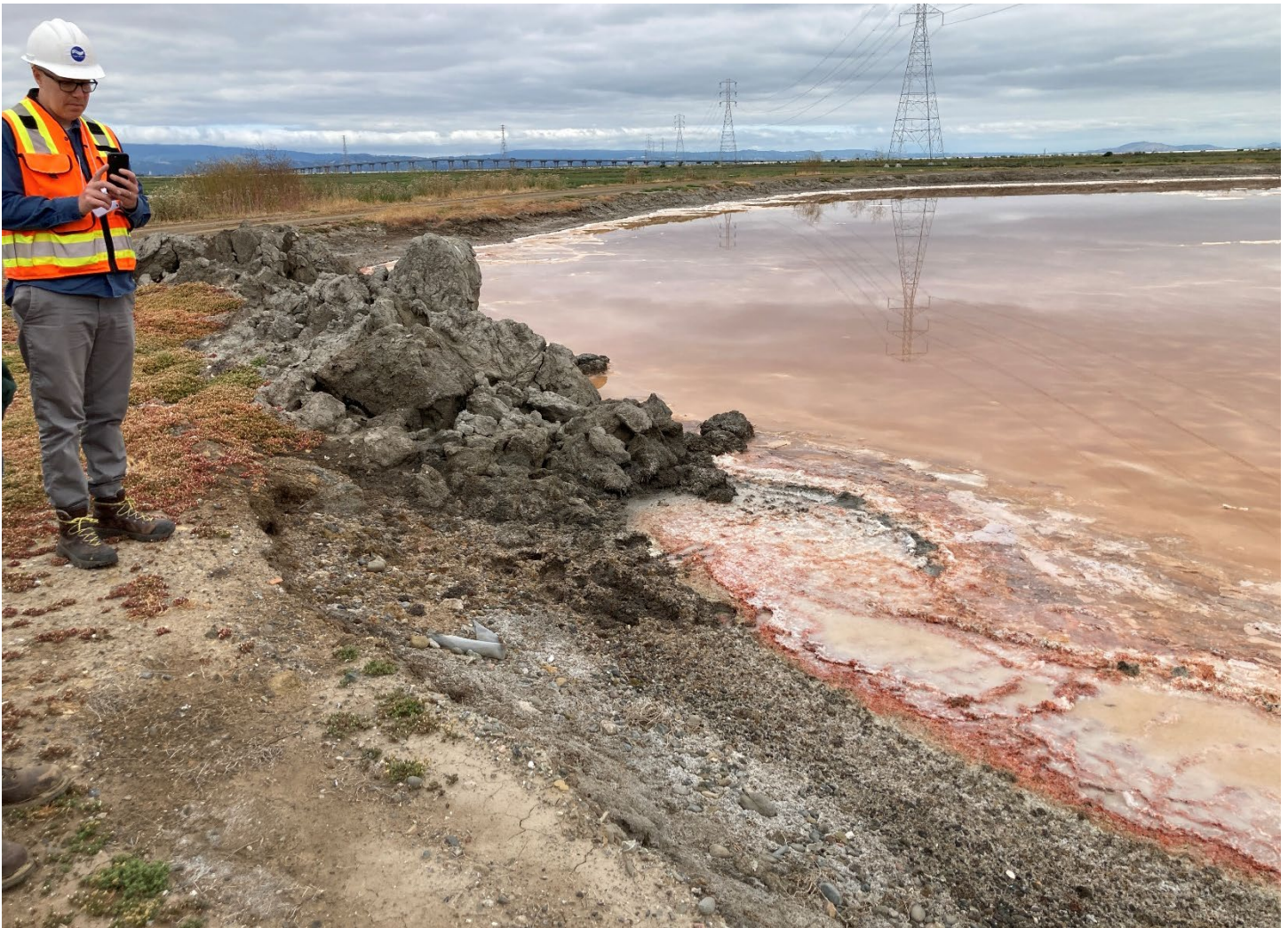
Photo 5. This photo shows the side cast from keying (berm coring) placed on the pond side of the berm at Pond P2-13. The pond has rainwater in it from the previous very rainy winter. The crystallized, solid mixed sea salts are visible at the edge and a few inches under the surface of the pond.
